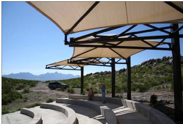
A beautiful new shade structure was installed above the Chihuahuan Desert Nature Park amphitheater in late August.
